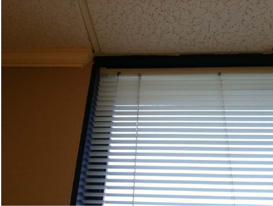
8 th Floor South – Farm Bureau – Head Detail: A.C.T. & Wood Trim painted, Walls: Painted GWB.
