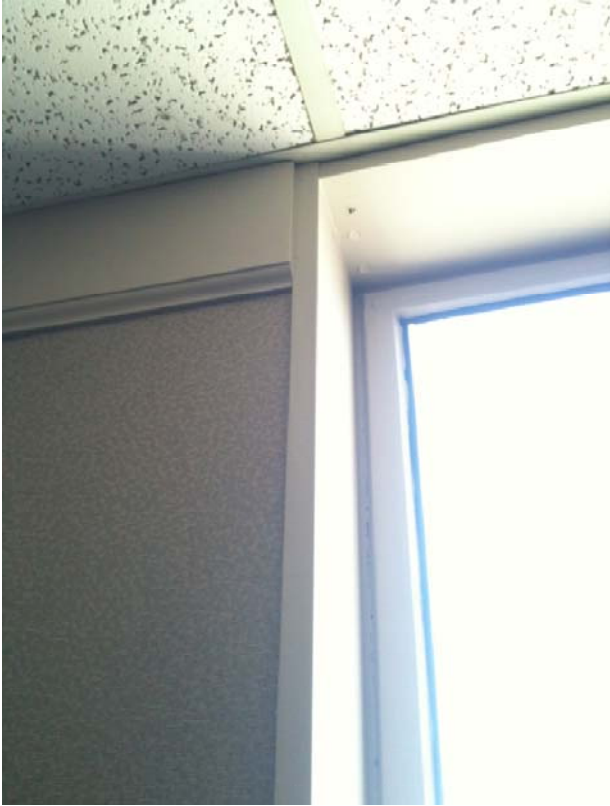
7 th South – Vacant Head Detail: Window Frame -painted; Wood trim –painted; A.C.T. ceilings
