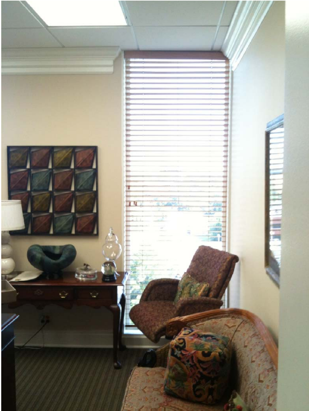
7 th Floor Window – Same as H & K windows on 6 th floor: Painted window frame, and painted wood trim.
