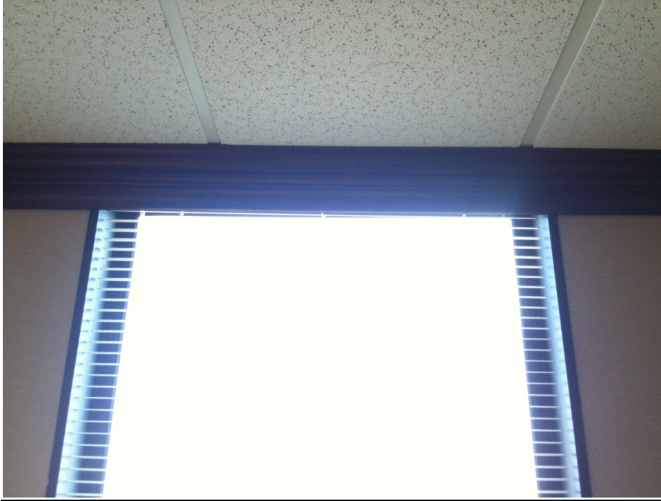
5 th Floor-Century Link Head Detail: A.C.T./Wood Crown Molding – window frame extends above/behind crown mold, metal blinds
