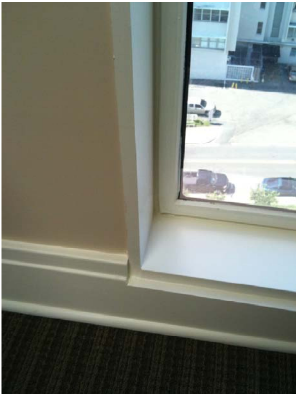
6 th Floor H&K Law Firm – Sill Detail: Wood Trim/Painted, Window Frame Painted;
