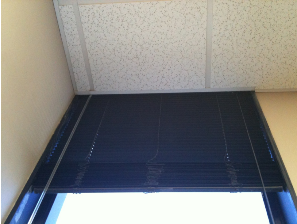
1 st Floor South – LC Supervisor of Elections – Head Detail: A.C.T. – Jamb: Painted GWB
